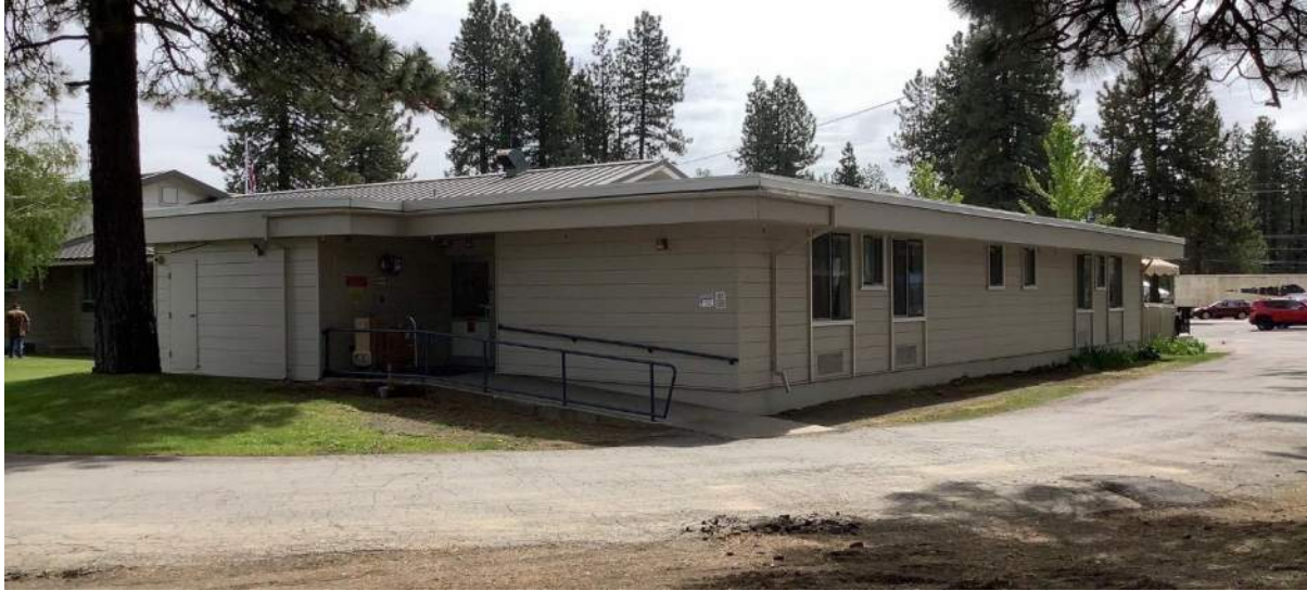
Figure 5-24. Overview of the north and west façades of the Extended Care Addition, view southeast.
